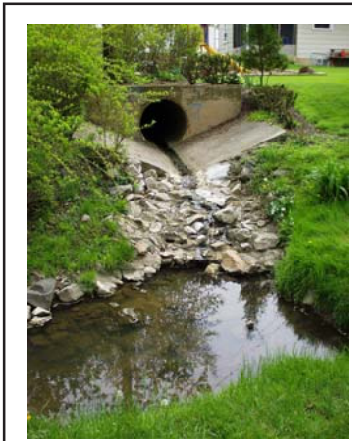
Storm drains wash pollutants straight into streams and lakes.
